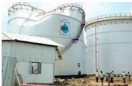
Figure 1. Tank Collapse Due to Accidentally Induced Internal Vacuum (de Paor 2010)
